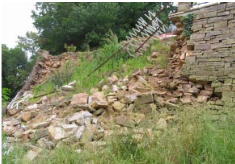
A section of the wall that we admired for so many years has tumbled down. Work is underway to replace this section and another that is also in danger of falling.
